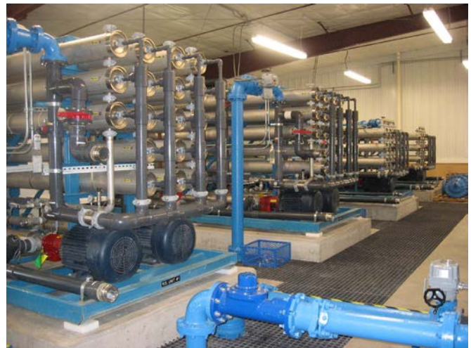
New Torrington WTP Showing Four RO skids
